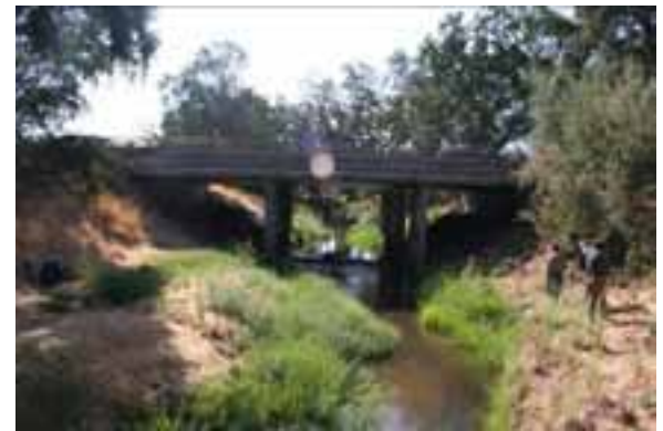
Old Auburn Road Bridge over Linda Creek, looking south at Crossing 28 site
