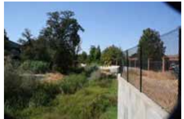
Maintenance ramp at bypass tunnel outlet (Crossing 14 site near Meadow Gate Drive access), looking west
