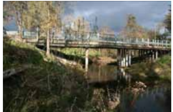
Existing Darling Way Bridge over Dry Creek may be used for path under-crossing
