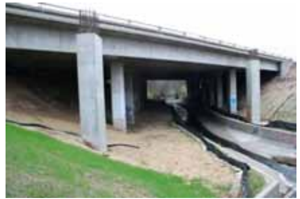
I-80 Bridge over Cirby Creek looking north (downstream); note 15' bench along left bank
